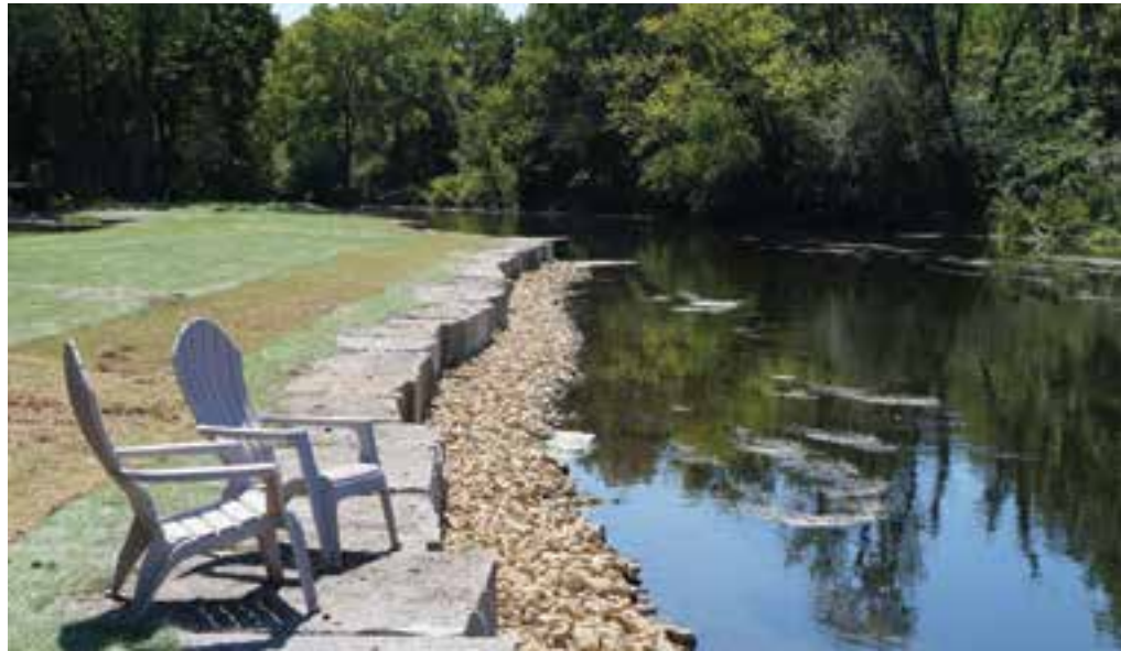
After construction of the ledge stone wall, residents were already enjoying their new backyard by placing chairs at the bank.
