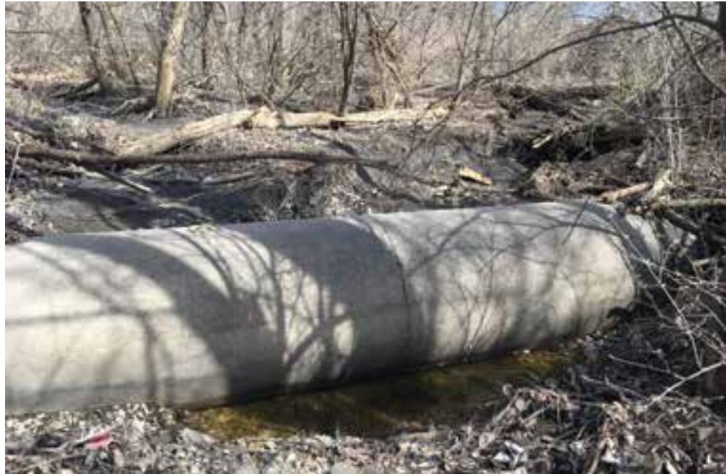
Exposed interceptor sewer pipe.
